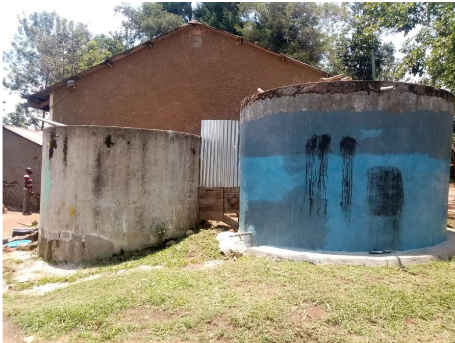
A water tank used that stores rain water used for irrigation
