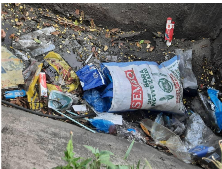
Drainage blockage by waste in Dar es Salaam
