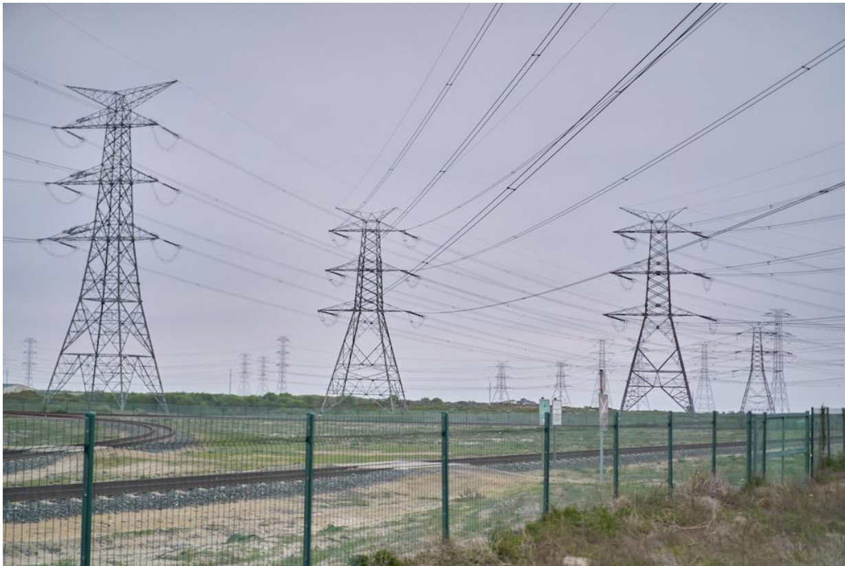
Atlantis transmits power to the national grid, in turn contributing to the creation of local jobs and locally-produced renewable energy. Photo: Barry Christianson
